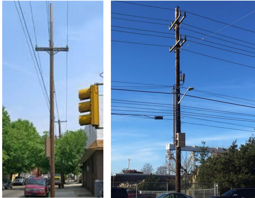
Cables and equipment are flush mounted and painted to match pole
