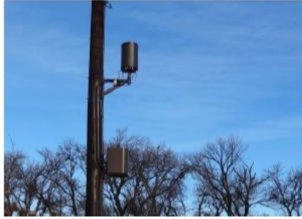
Cables are flush mounted and all equipment is painted to match pole
