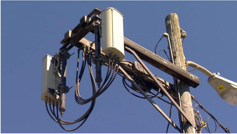
Exposed cables and antennas not painted to match pole
