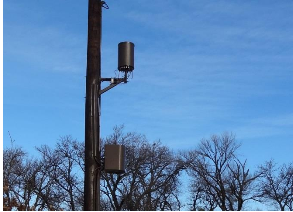
Cables are flush mounted and all equipment is painted to match pole
