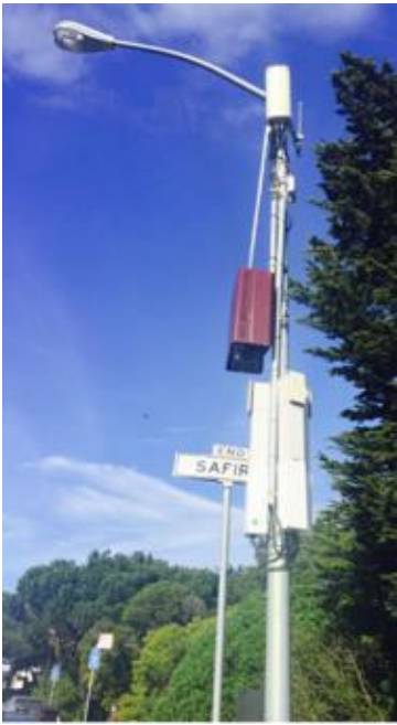
Exposed slack on cables and bulky equipment
