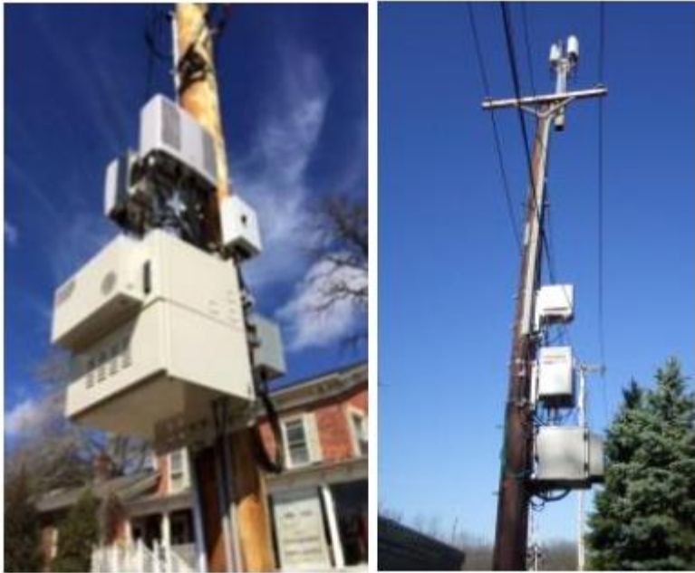
Bulky equipment not flush mounted or painted to match pole
