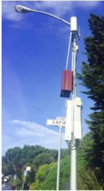
Exposed slack on cables and bulky equipment
