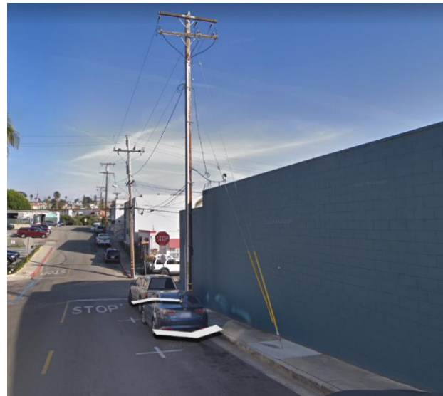
Allowed on utility poles extending above adjacent buildings
