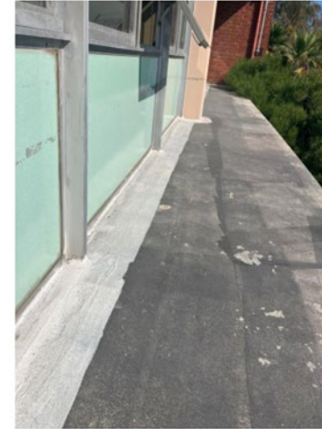
Second floor windows leak
