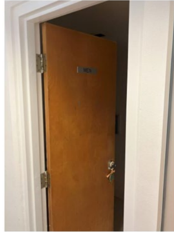
Restroom doors need sound proofing
