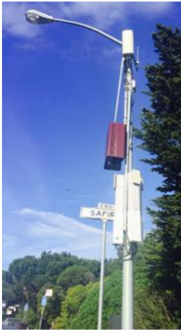
Exposed slack on cables and bulky equipment
