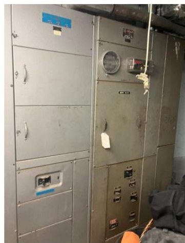
Electrical panels need to be upgraded
