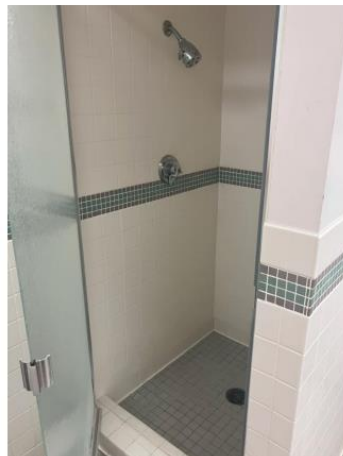
Bathroom needs upgrades
