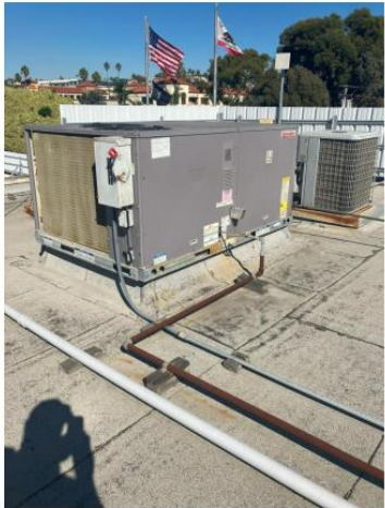
A/C Units and roofing
