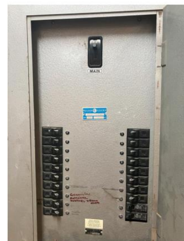
Electrical panels need to be upgraded
