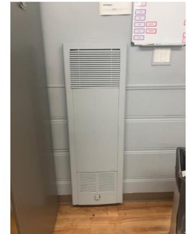
No heating throughout building
