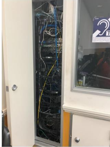
Old electrical wires
