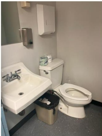
All plumbing backing up constantly
