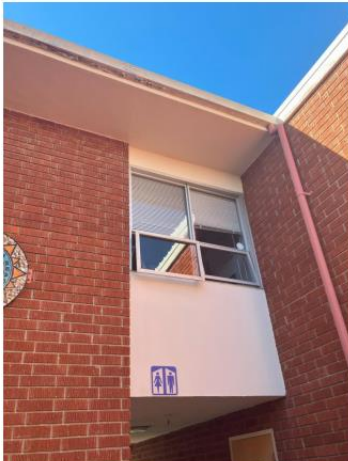
Windows (framing is old and damaged) Page 6
