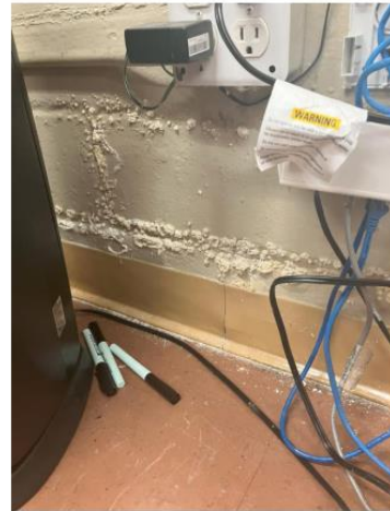
Mold on northeast wall (interior)
