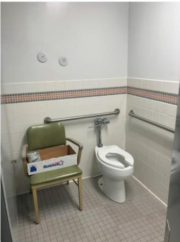
All plumbing backing up constantly
