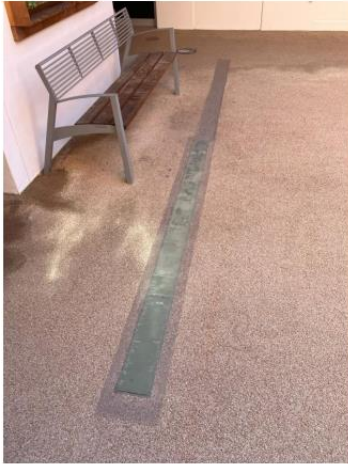
Crack under courtyard leaks into basement and IT room
