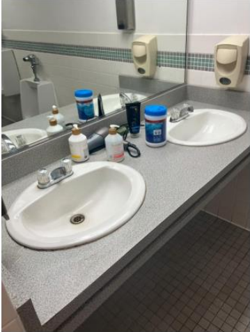
Bathroom needs upgrades
