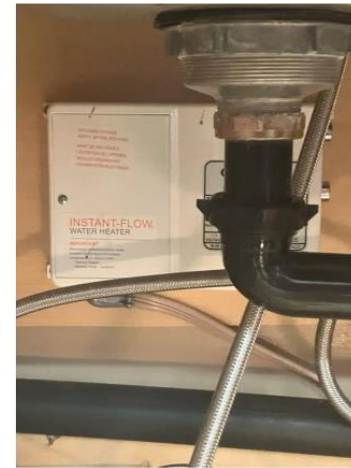
No hot water (water heater needed)
