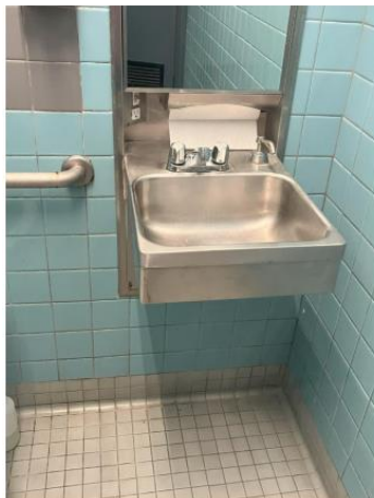
Bathroom needs upgrades
