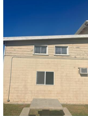
Windows leaking and damaged
