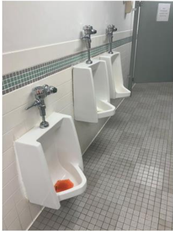
All plumbing backing up constantly
