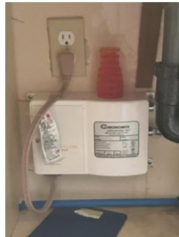
No hot water (water heater needed)
