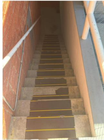
Gutters leak onto stairway
