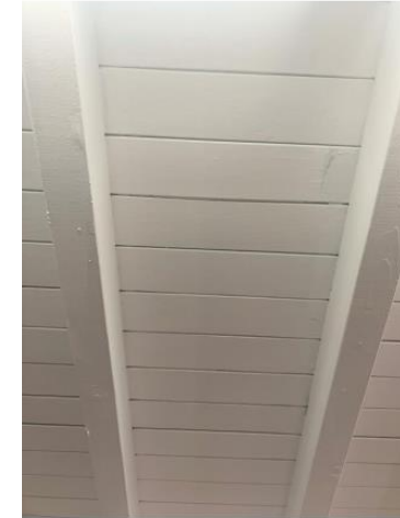
Termites on roof
