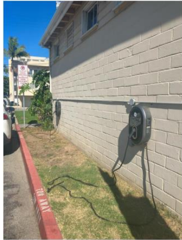
Electric Vehicle Charger (westside wall)
