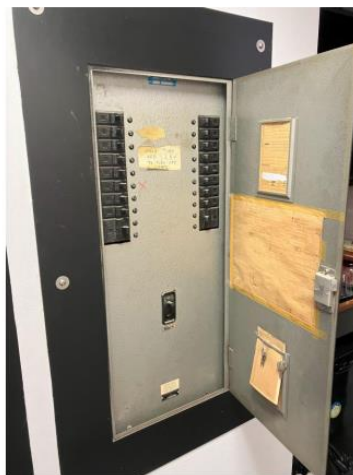
Old electrical panel needs to be upgraded
