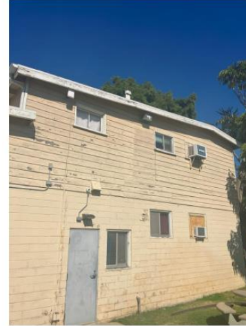
Air conditioning units
