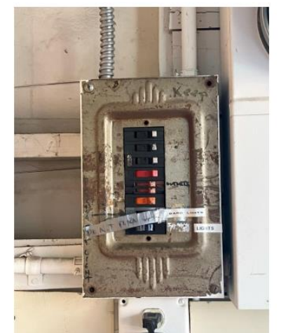
Old electrical panel
