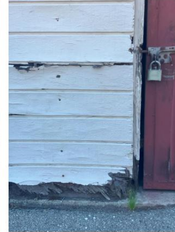
Water damage and wood rot
