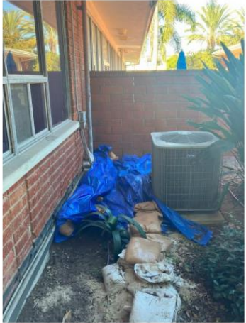
Leaking into Men's Locker
