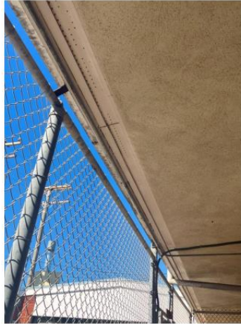
Gutters leak onto stairway
