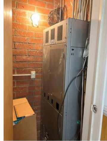
Old electrical wires
