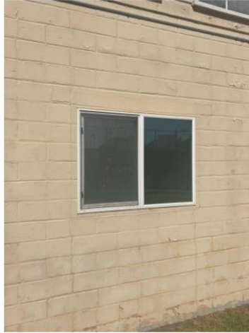
Windows leaking and damaged
