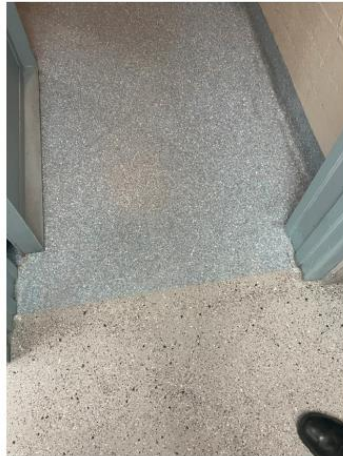
Leaking into Men's locker room
