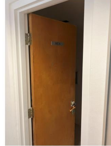
Restroom doors need sound proofing
