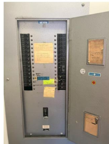
Old electrical panel needs to be upgraded Page 7
