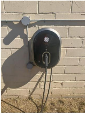
Electric Vehicle Charger (westside wall)
