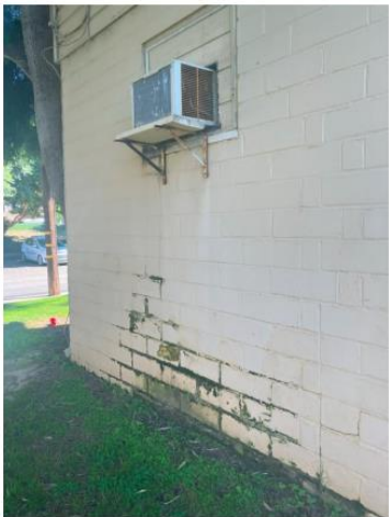
Mold on northeast wall (exterior)
