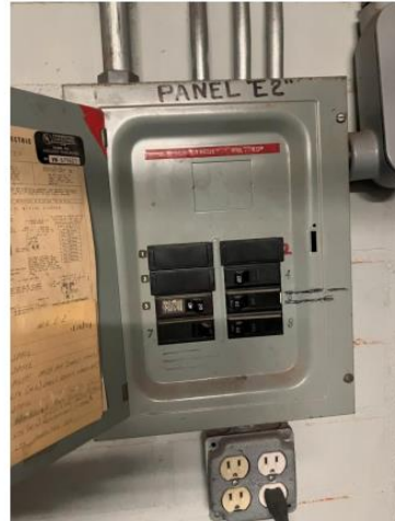
Electrical panels need to be upgraded
