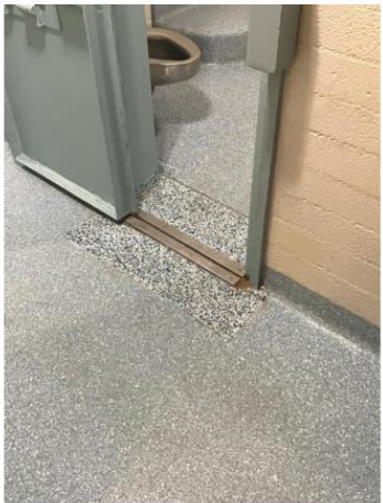
Leaking into Men's locker room
